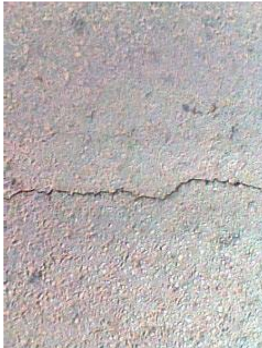
Plate 2. Failed portion of the intra campus Road, University of Agriculture, Makurdi, Benue State, Nigeria.
