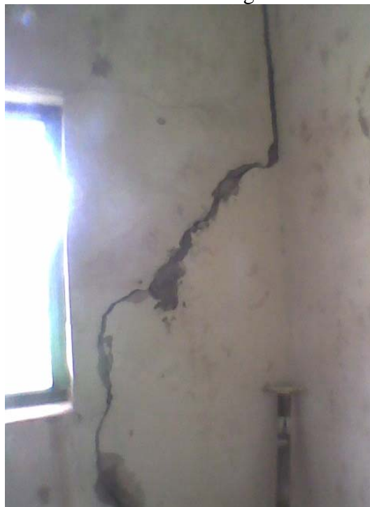
Plate 1. Cracks on Building founded on shale deposits located at the College of Engineering, University of Agriculture, Makurdi, Benue State, Nigeria.
